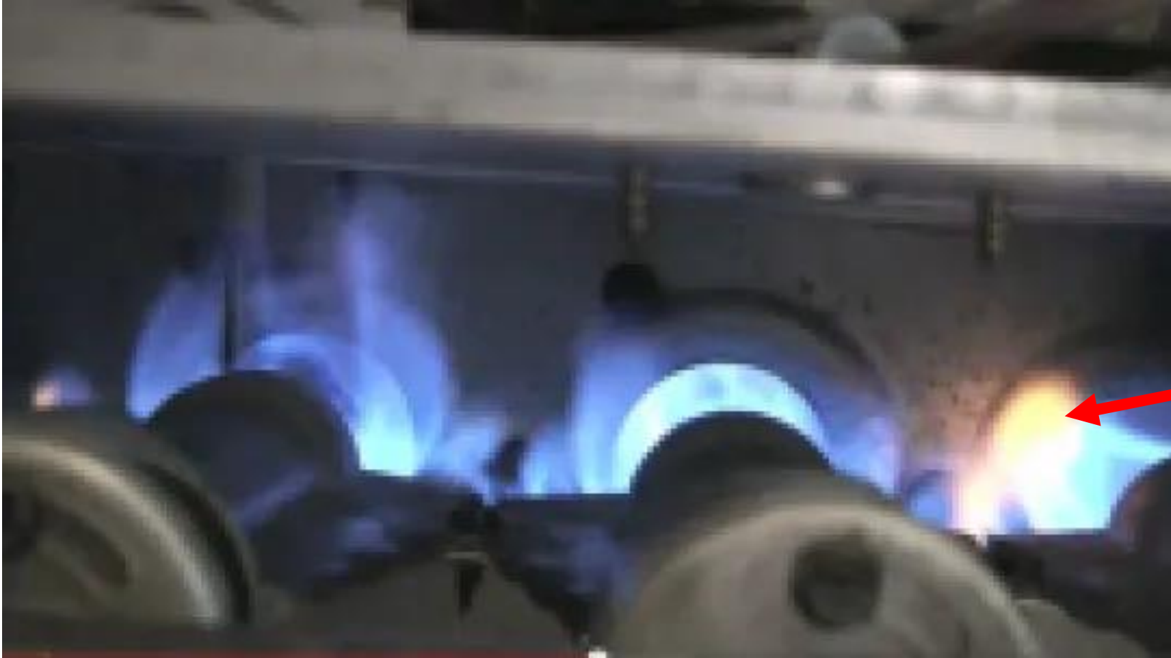
Potential Cracked Heat Exchanger
