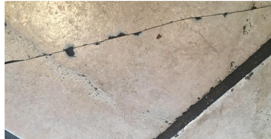
Cracked Floor Tiles
