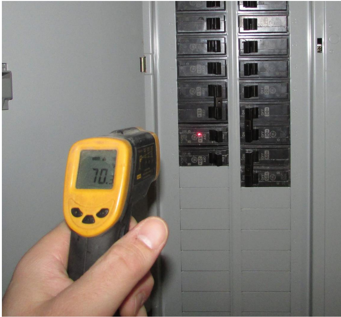
Breaker Temperature Reading
