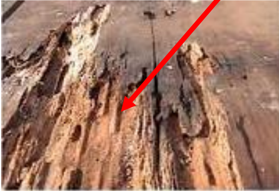
Termite Damage (with grain)
